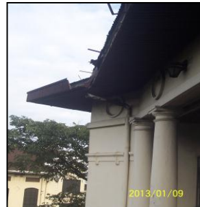
Plate No.4 Dilapidated roofing at the 4 th floor. It was destroyed by Typhoon Yoling in 1970.
