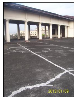
Plate No.5 Caracks at the rooftop caused by time, rains and earthquakes
