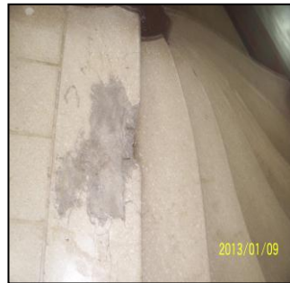
Plate No. 6 Evident cracks in the stairs.
